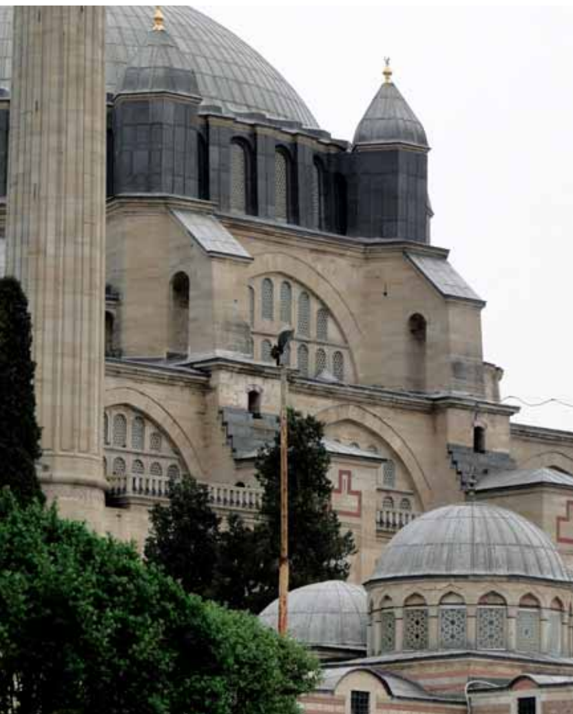
Fig. 83: Southwest elevation, cascading buttresses and weight towers around the base of the main dome.
